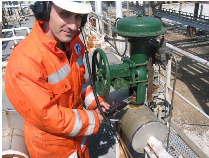
Internal Leak Detection with the PS-2100 in an LPG Valve
